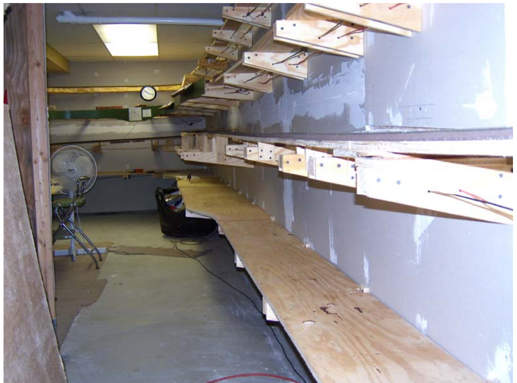
Overview of the new bench work for the Merced staging yard. At the end of the room two decks above the SP staging is the town of Tuolumne, the end of the line for the Sierra.
