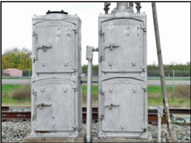
Cases hold relays for the signal logic at Fairmead.
