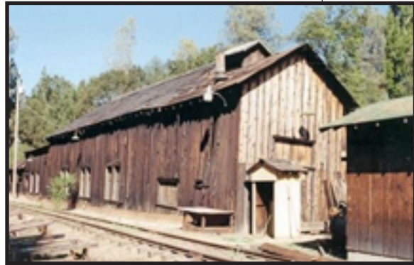
Look at the knots on the ends of this building. Also look at the weathering towards the bottom of the foreground building.
