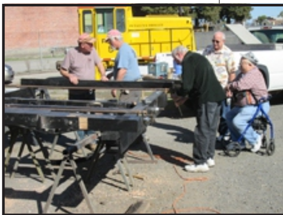
RED members watch while a new wood beam is being installed on a set of trucks.
