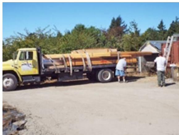
On 7-17-15 this truck arrived beside the prepared ground with everything except the concrete needed for the construction of Gus' officially large garage and shop.
