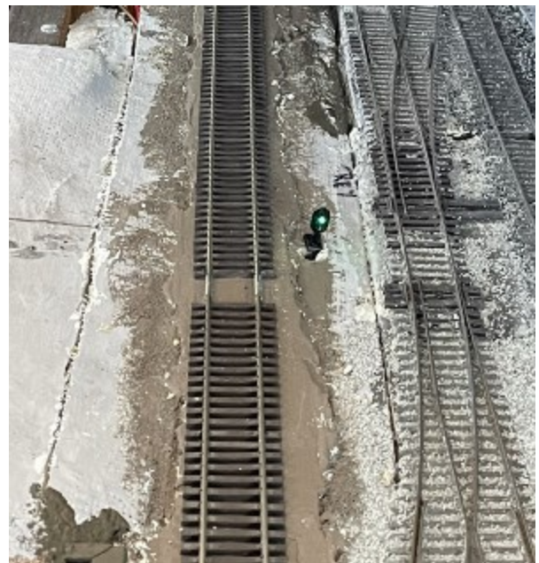
Figure 6: Entry track on left from ENL into the loop, showing protecting dwarf signal.
