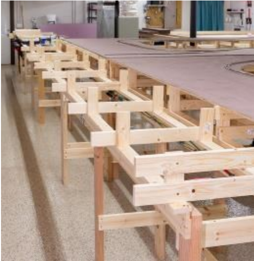
Risers have been installed for the first 16 feet of the 32' total for the Cloud's Rest yard. Plywood support joists will be added and then topped with plywood.
