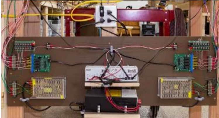
A Digitrax power supply providing DCC power to two of the three PM42 units which supply power to 8 of the 12 sub-districts. Also visible are two additional 12-volt DC power supplies.
