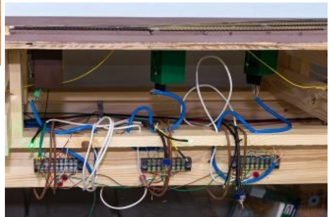
Two SMAILs and one Tortoise by Circuitron switch machines are wired with toggle switches and LED panel indicator lamps. The SMAILs are DCC enabled and can be controlled from a throttle, by the attached toggle switches and via JMRI.
