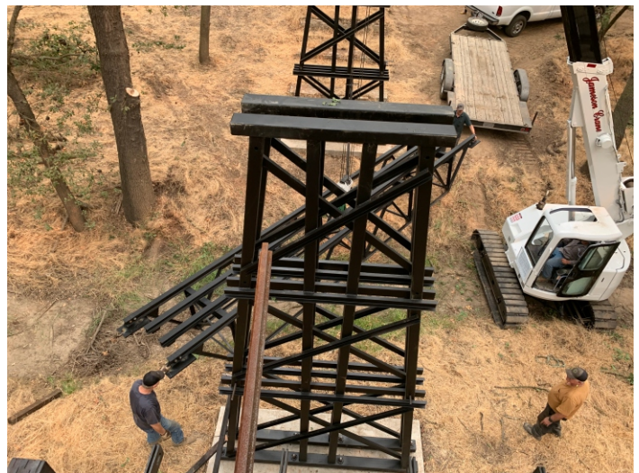
Recent construction activity on the Hillcrest & Wahtoke RR saw the erection of a trestle across Wahtoke Creek.
